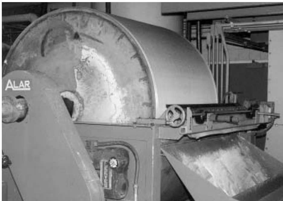
An Auto-Vac Filtration and De-watering System has been modified to handle fine alum sludge generated by the Tewksbury, Mass., water treatment plant.
